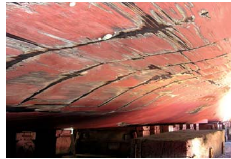
Bottom damages as a consequence of machinery failures 1
