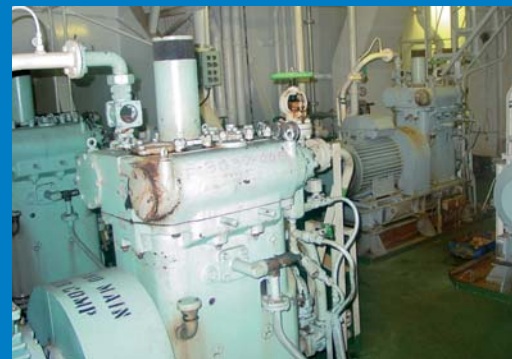
Typical air compressors on a vessel
